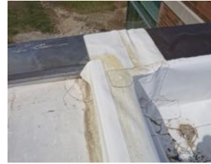
This coping intersection was never properly detailed, and roofed over with white tape and contact cement.
