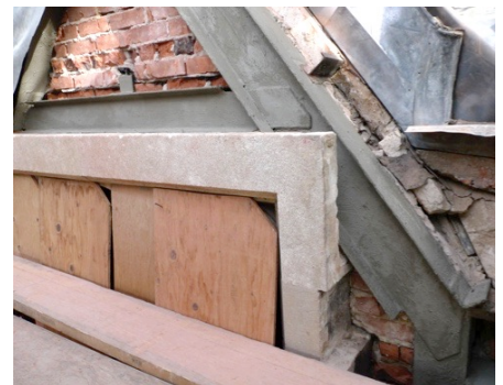
Severely rusted steel was uncovered, painted with a cementitious alkaline coating, and then cathodically protected from future corrosion.
