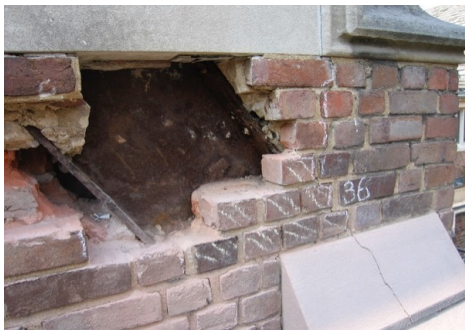
Cracks through the masonry originated at the flanges of steel beams
