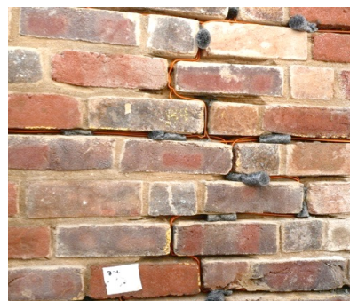
Titanium and ceramic anodes, drilled into the wall at pre-set locations, were connected to their power source by titanium wires embedded in mortar joints.
